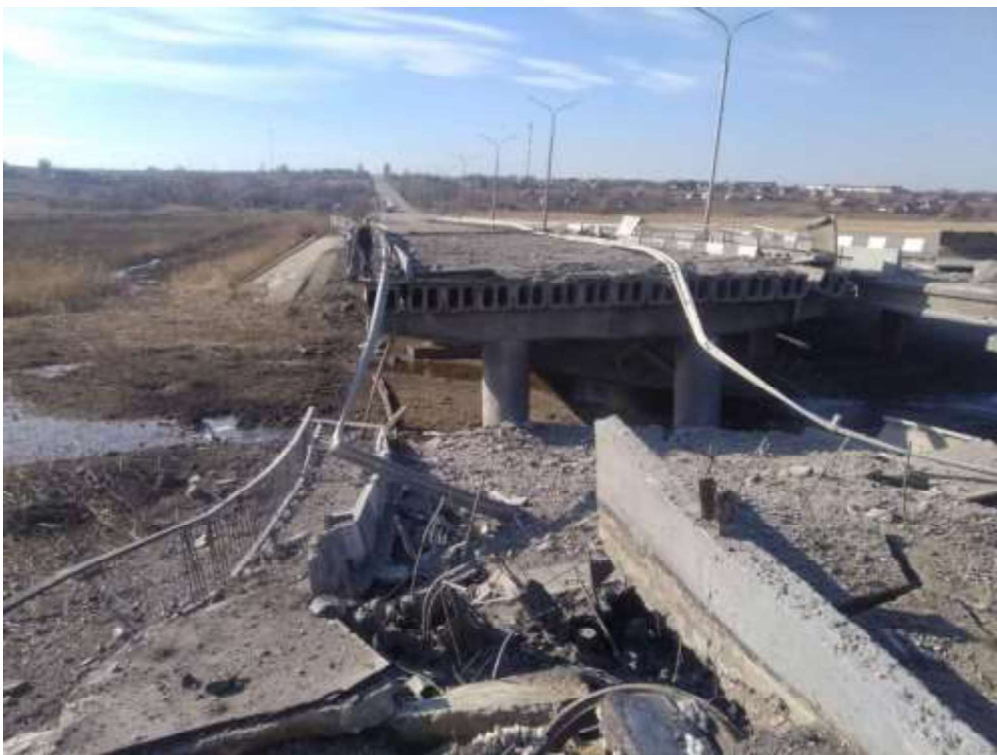
A ruined bridge through the village of Kamianske
