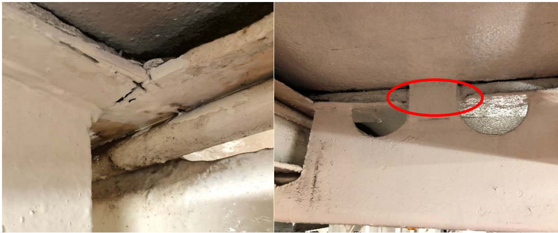
Figure 14 - Typical details of cut outs: intersection of stiffener and frame (left), web frame with plate missing (right)
