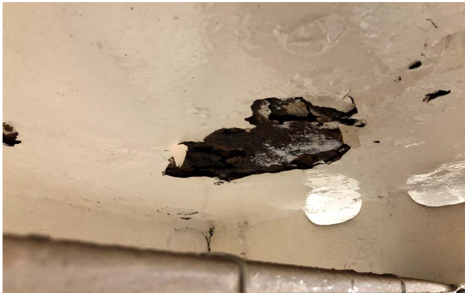
Figure 4 - Typical state of original deck plating, with irregularities and holes
