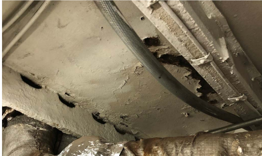
Figure 3 - Example of poor condition of coating below original deck plating
