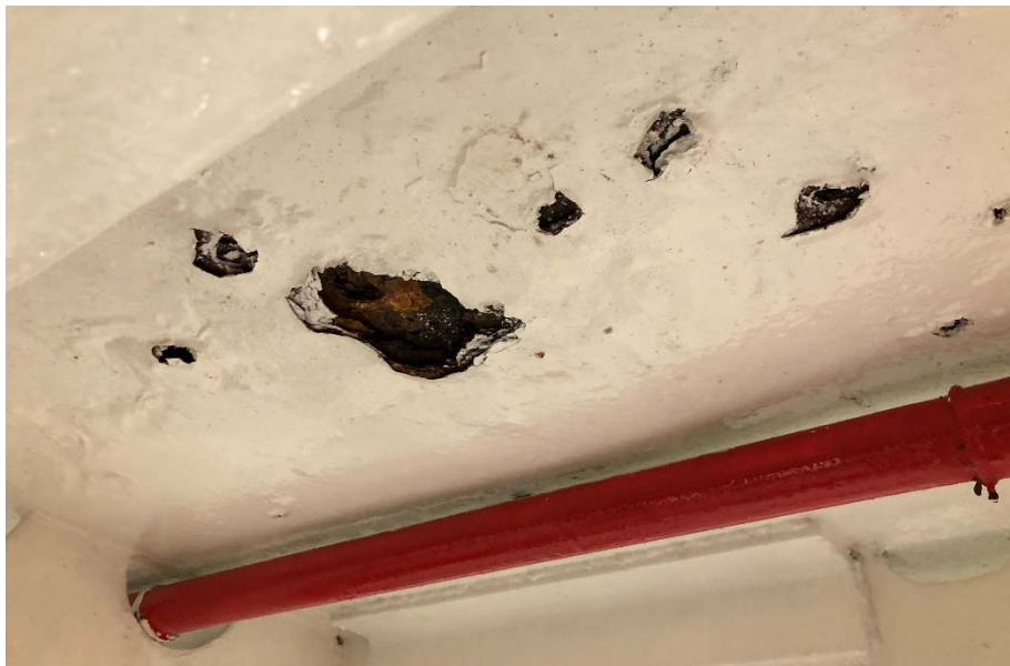
Figure 5 - Original deck plate field with multiple holes and flaking of steel plate
