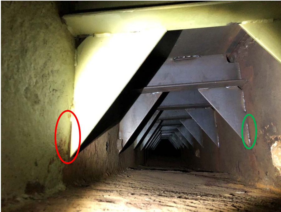
Figure 33 - Example of brackets inside old cooling water tank, with missing weld at ends (red)
