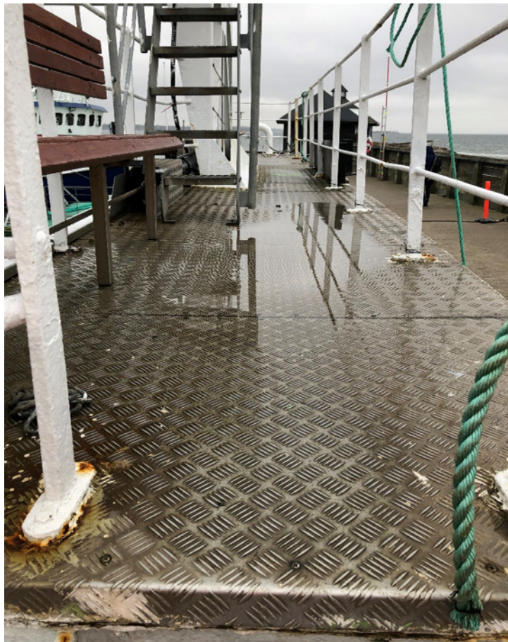
Figure 25 - Passenger platform, presenting poor drainage
