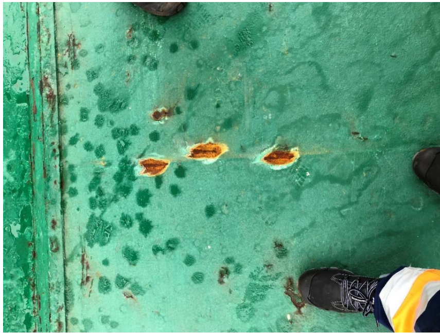
Figure 11 - Failure of coating system in way of slot welds
