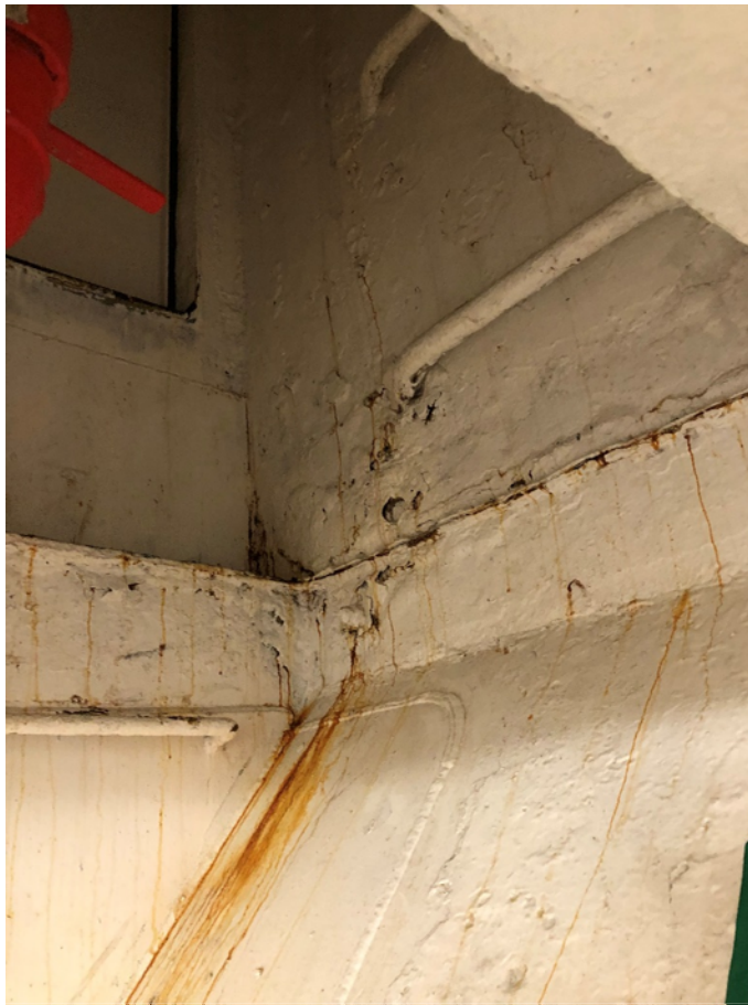
Figure 20 - Corrosion hidden under coating, in way of Engine room emergency exit
