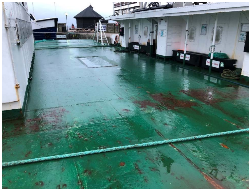
Figure 10 - Condition of top deck plating
